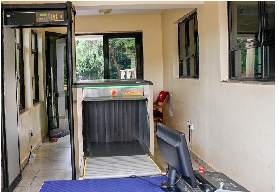
The Security system installed at the entrance of KSG Lower Kabete to ensure the security of KSG staff, participants and clients. It is inclusive of; a metal detector used to identify concealed weapons such as guns or knives and an xray machine used for screening luggage. Qualified security personnel have been deployed at the gate to ensure that persons accessing the School are taken through the necessary checks to ensure security for all.
